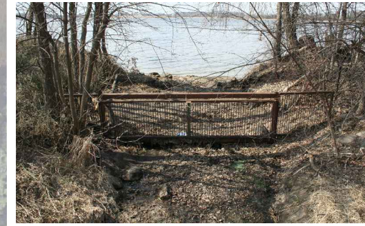
PHOTO D. FISH BARRIER INSTALLATION EXAMPLE 2
