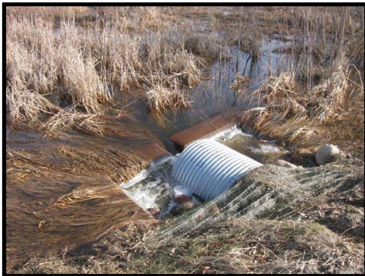
Photo 3-Clear Lake V-notch Weir
