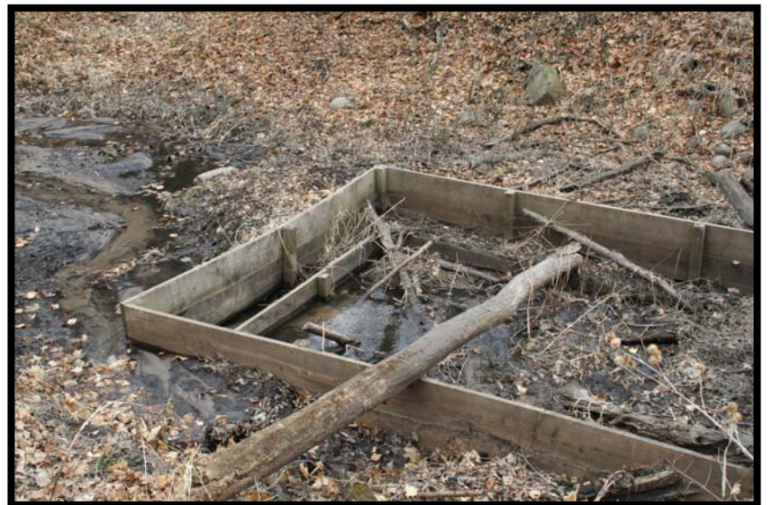
Photo 12-Lake Augusta Sedimentation Pond Inlet Box
