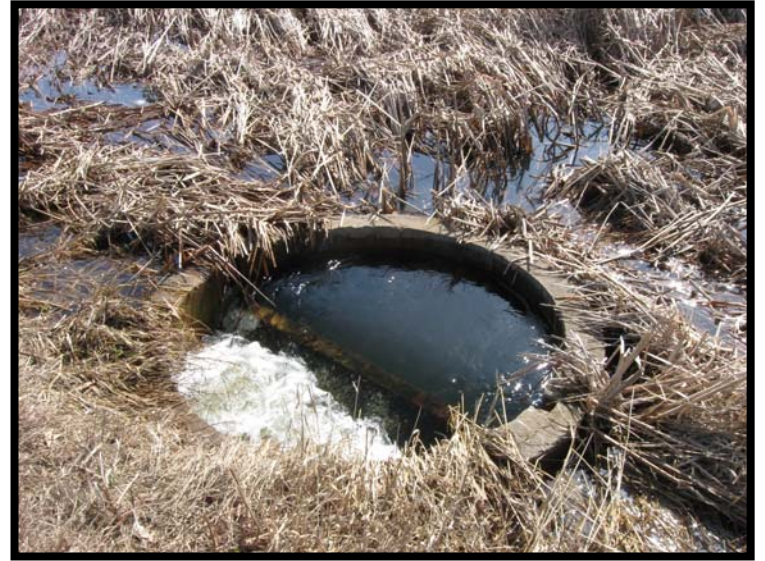
Photo 10-Annandale Wetland Diversion Structure
