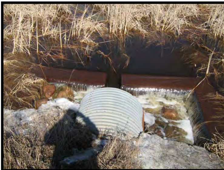
Photo 3-Clear Lake V-notch Weir.
