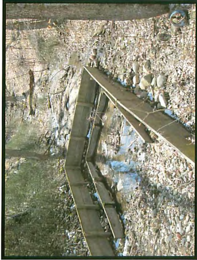
Photo 29-Lake Augusta Erosion Control Project Sedimentation Box (West)
