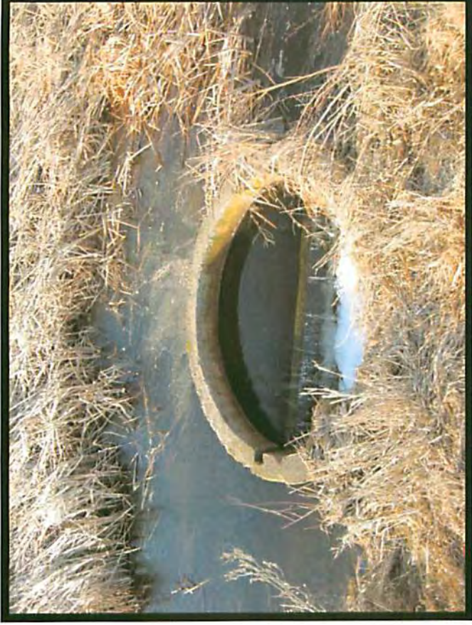
Photo 22-Annandale Wetland Treatment System Outlet Structure
