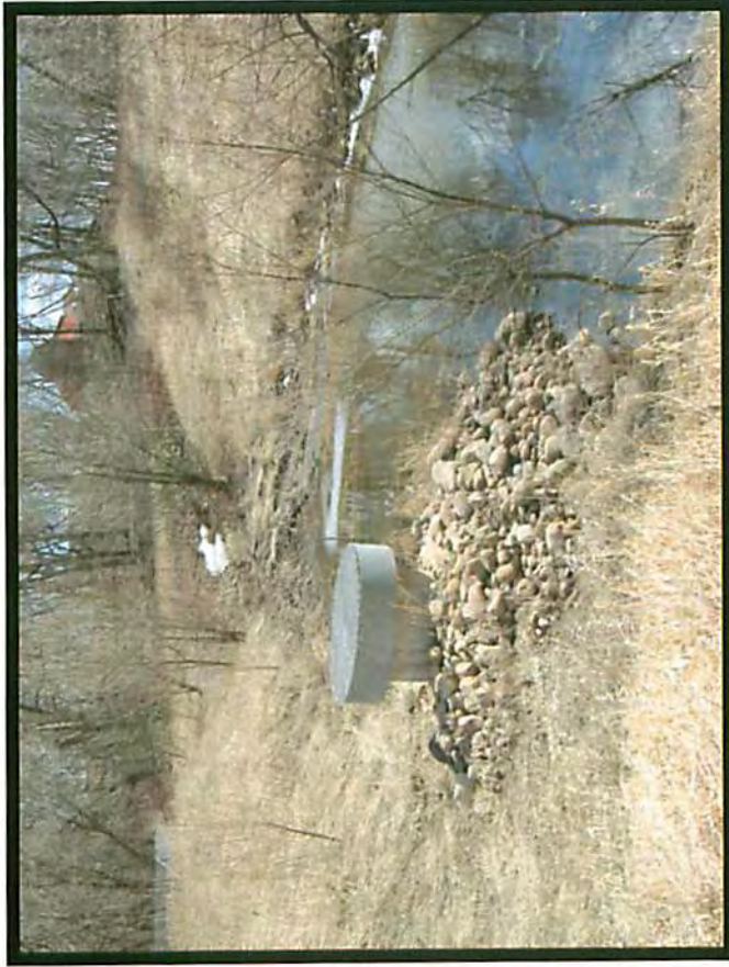
Photo 31-Lake Augusta Erosion Control System Riser (Cracks in bottom of structure to be repaired in 2007)
