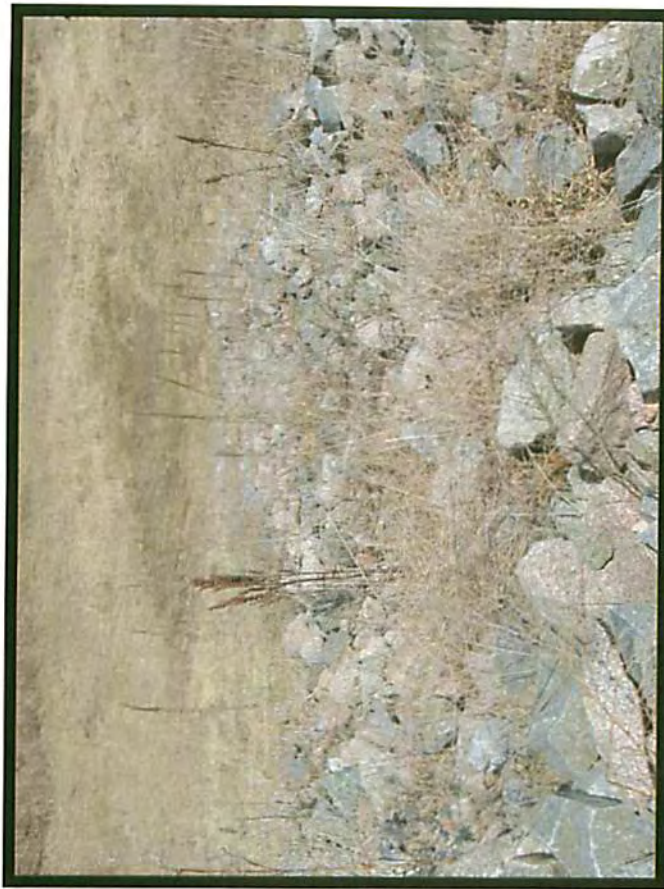
Photo 14-Rest-a-while Sedimentation Basin (East)
