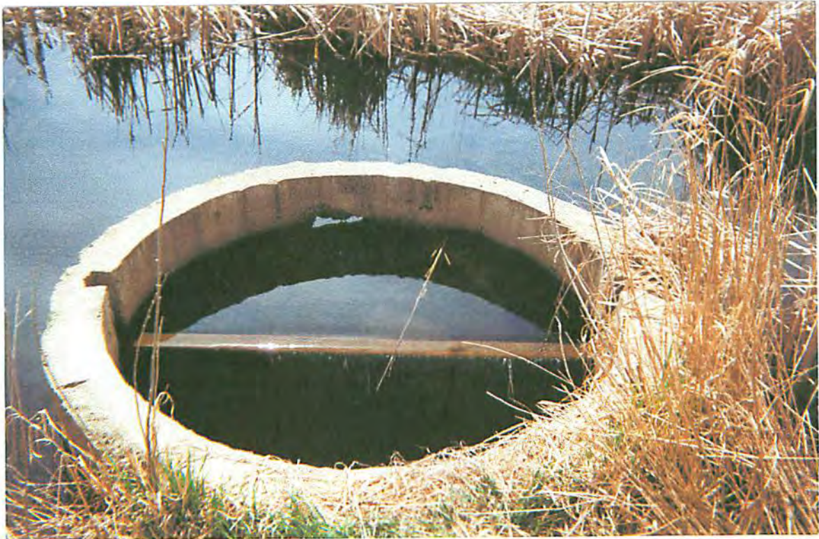
2. Annandale Wetland Treatment Project Control, Outlet Structure.
