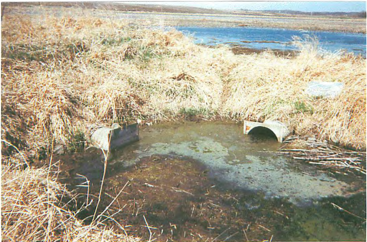
4. Upper Watkins Wetland Isolation Project. North Ditch Controls.
