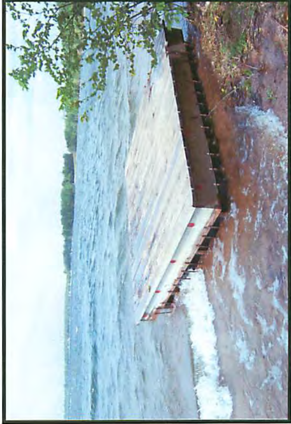
Photograph 7: Pleasant Lake – outlet structure.
