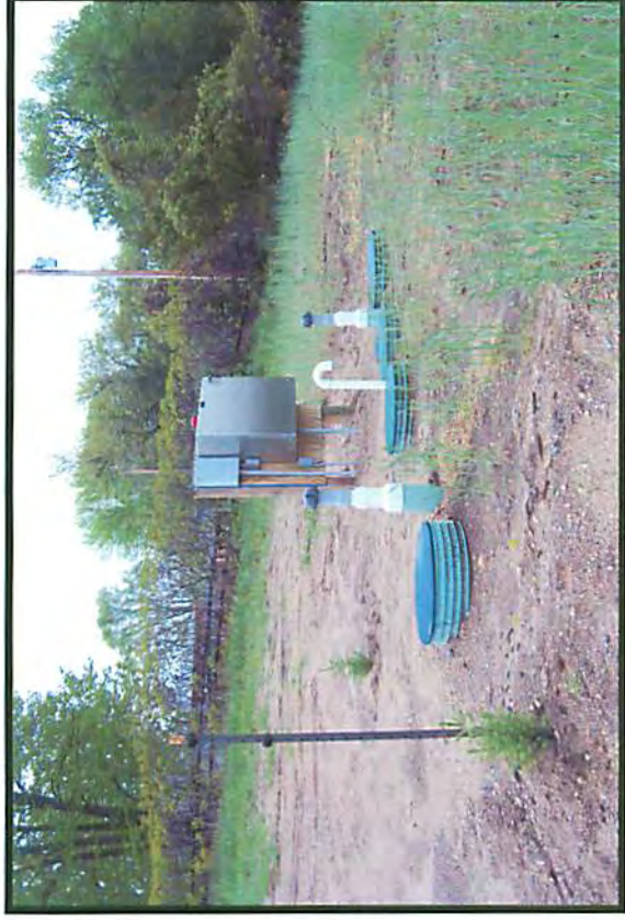
Photograph 18: Rest A While Sewage Treatment Facility.
