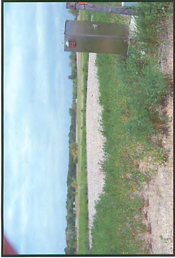
Photograph 17: Hidden River Sewage Treatment Facility.
