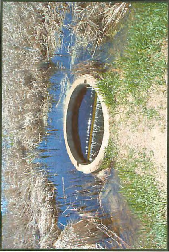
Photograph 5: Annandale Wetland – Outlet Structure
