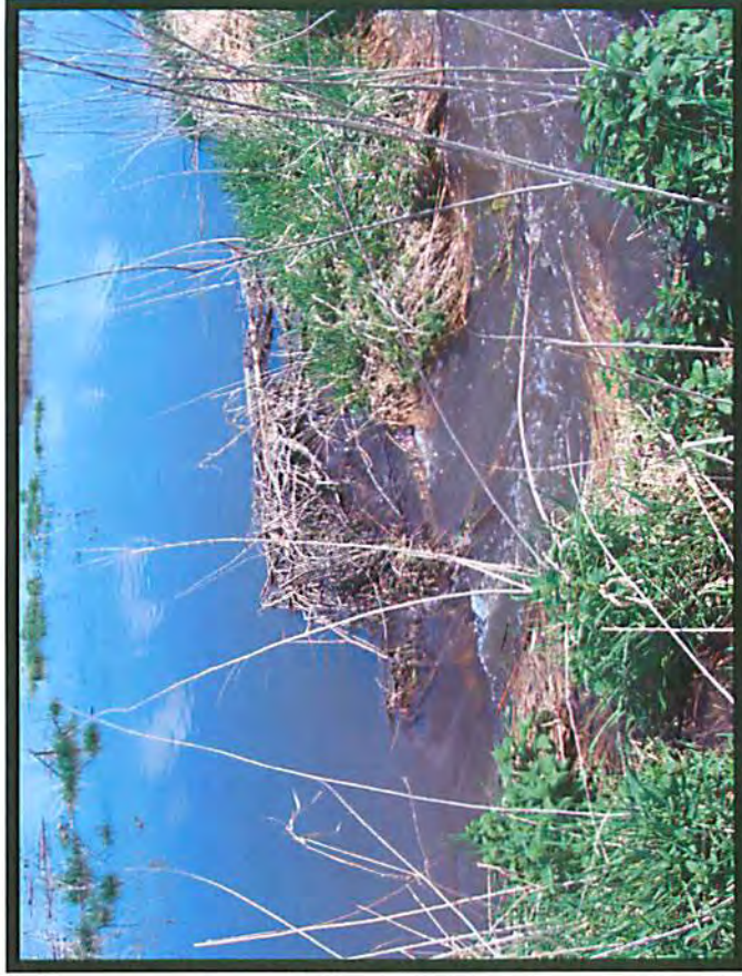
Photo 12 Kingston Wetland Treatment System – Berm washout
