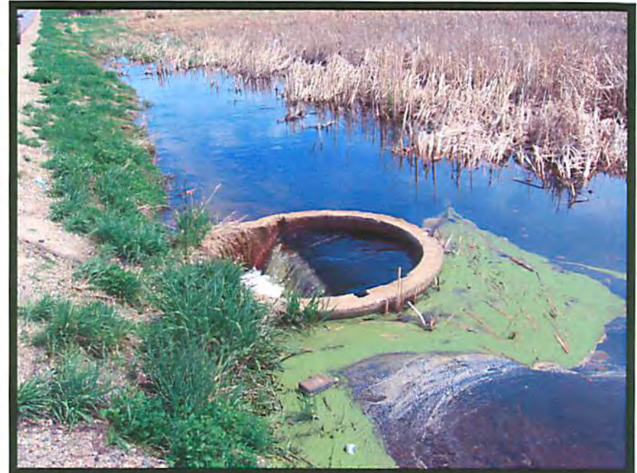
Photo 26 Annandale Wetland Treatment System Outlet Structure
