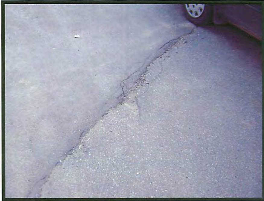
Photo 23 Clearwater Harbor Wastewater Collection and Treatment System (Blacktop Seam)
