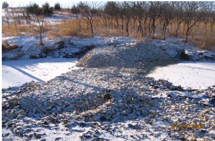
A diversion berm was constructed in December 2007 to divert stream flow into Segner Pond, a sedimentation basin on the Cedar Lake inlet.
